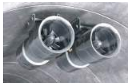
Wentylatory w tunelach
